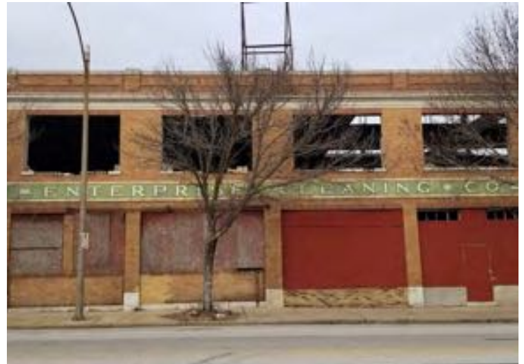
Vacant storefronts sit unoccupied and abandoned on a commercial corridor
